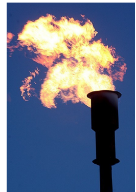
Because of the gas utilization project, the flare to burn off landfill gas is no longer active
