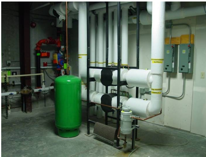
Standard Imaging's geothermal pump utility room
